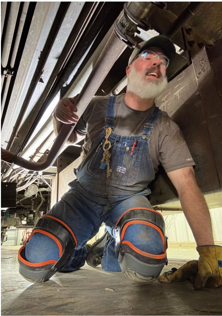
Volunteer Paul Stephens assists Eric Dilbeck with installing power cables under our 115 passenger coach for Head End Power.
