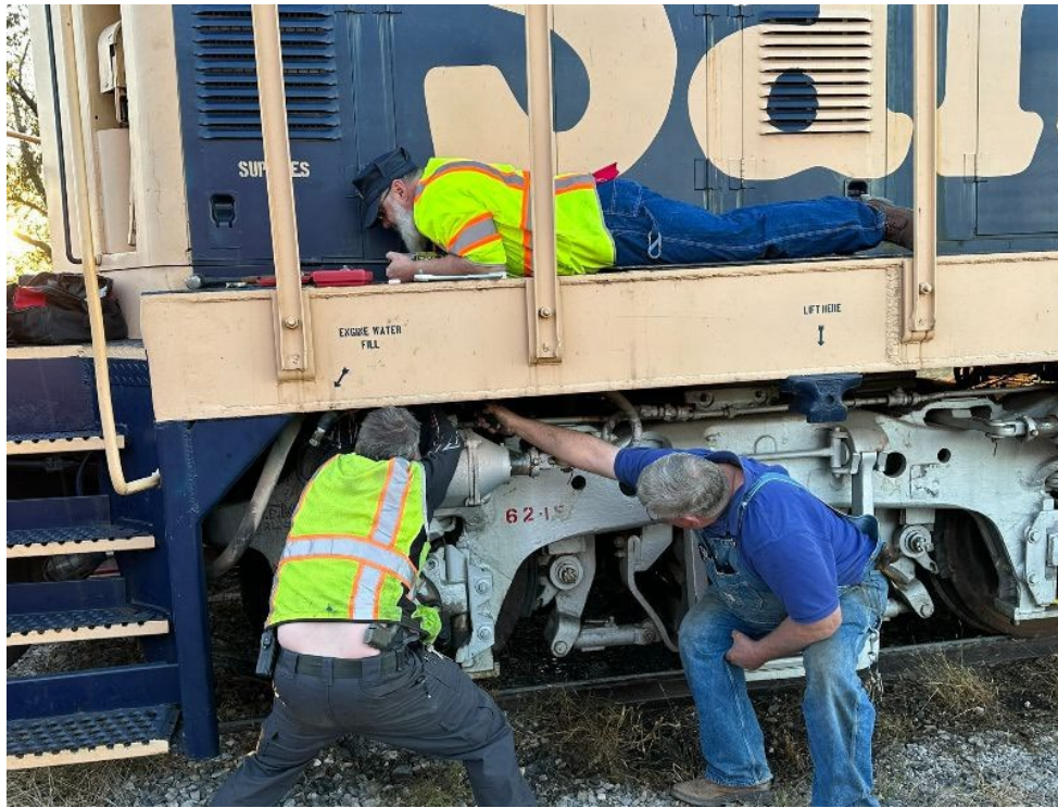
John Nave and Greg Hall(L-R) is assisted by Paul Stephens above on repairing a air leak on the Santa Fe CF-7.This was during the tech rehearsal for Polar Express.
