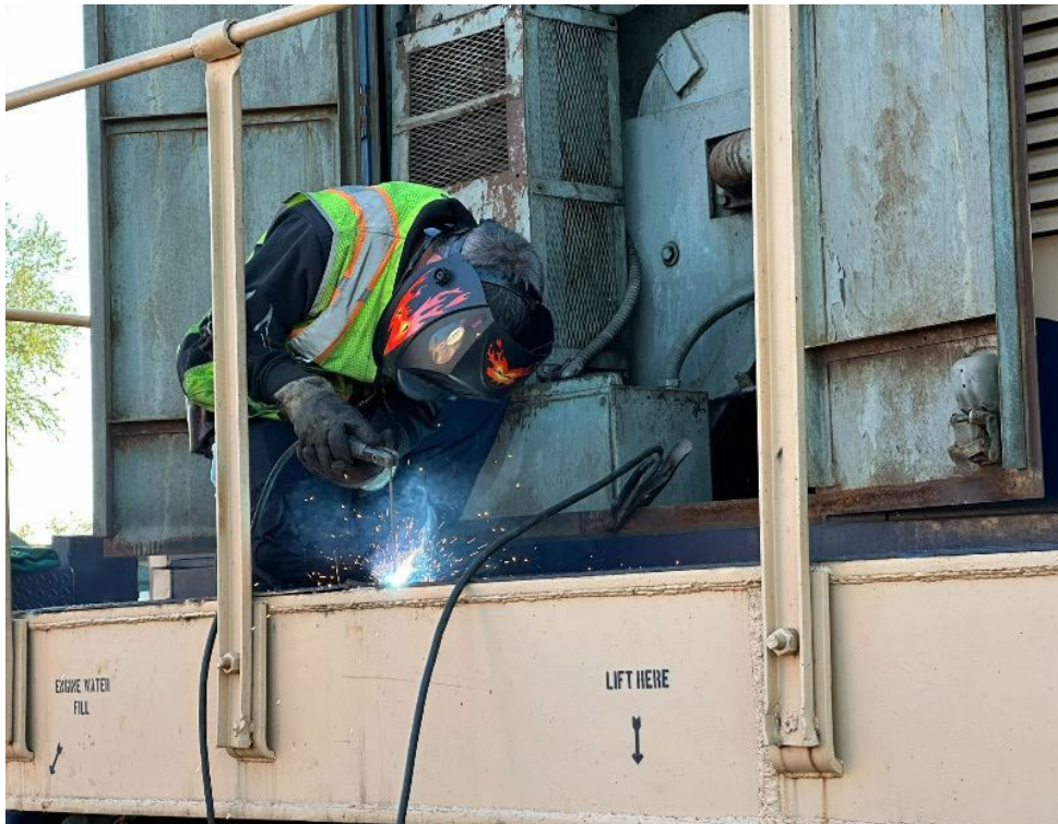
Vice President John Nave is busy welding up a deck plate that was removed to repair a air leak on the CF-7.
