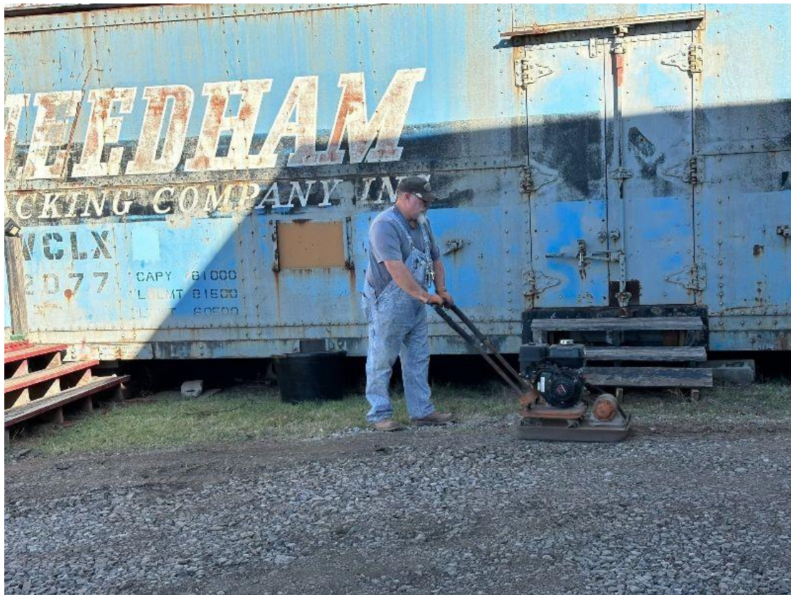
Jay Chilton works on packing our drive that goes along the side on the Jim Murry Maintenance Facility. Jay also repaired the drainage in the area due to damage from trucks driving through to the back of the shop.
