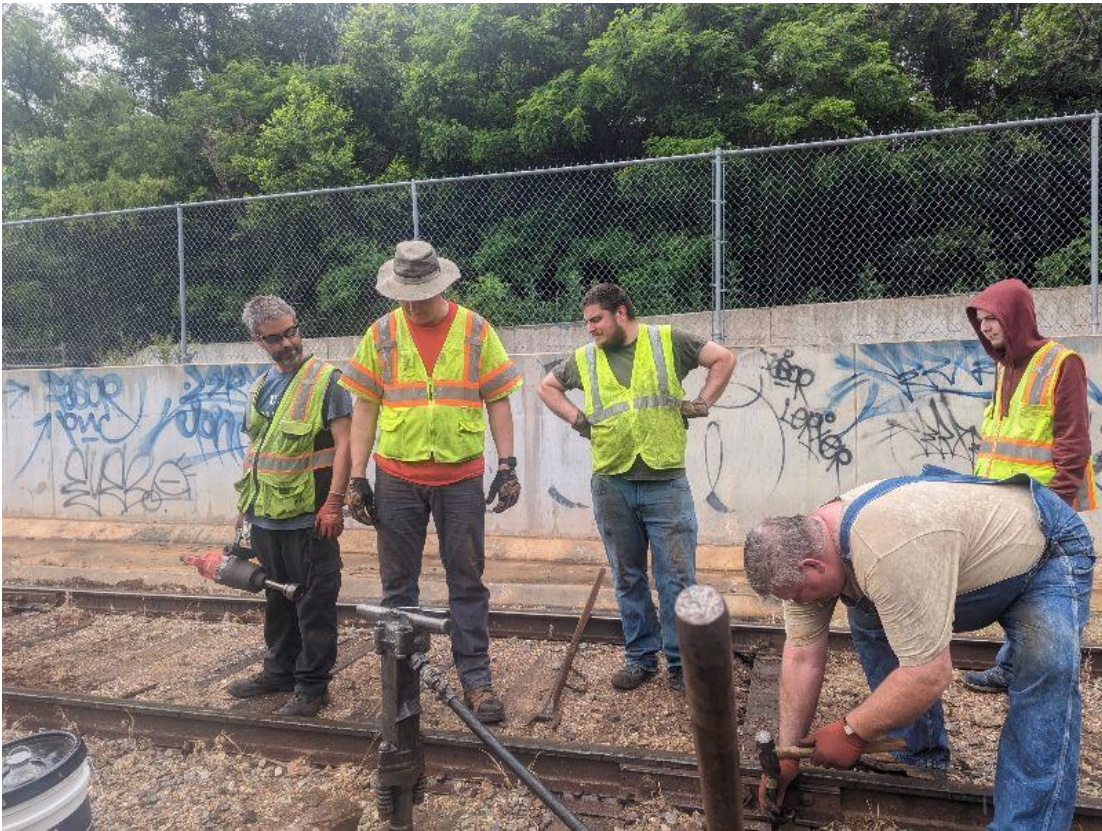
Our track crew replaced 12 ties just south of the 23rd street underpass on Memorial day May 29th. Volunteers pictured: (L-R) John Nave, Eric Dilbeck, Kevin Oakley, Greg Hall and Clayton Nave. Not pictured was Andrew Reynolds, Caleb Nave, and Natalie Lawson.
