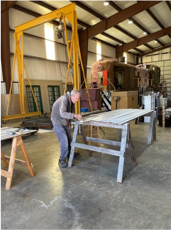
Volunteer Charles Prices paints boards for the interior of Le Flore Depot
